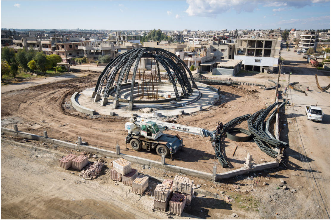
Construction of the new parliament and surrounding park in the city of Derik in the autonomous region of Rojava on 5 December 2015. Photo: Ruben Hamelink, New World Summit
